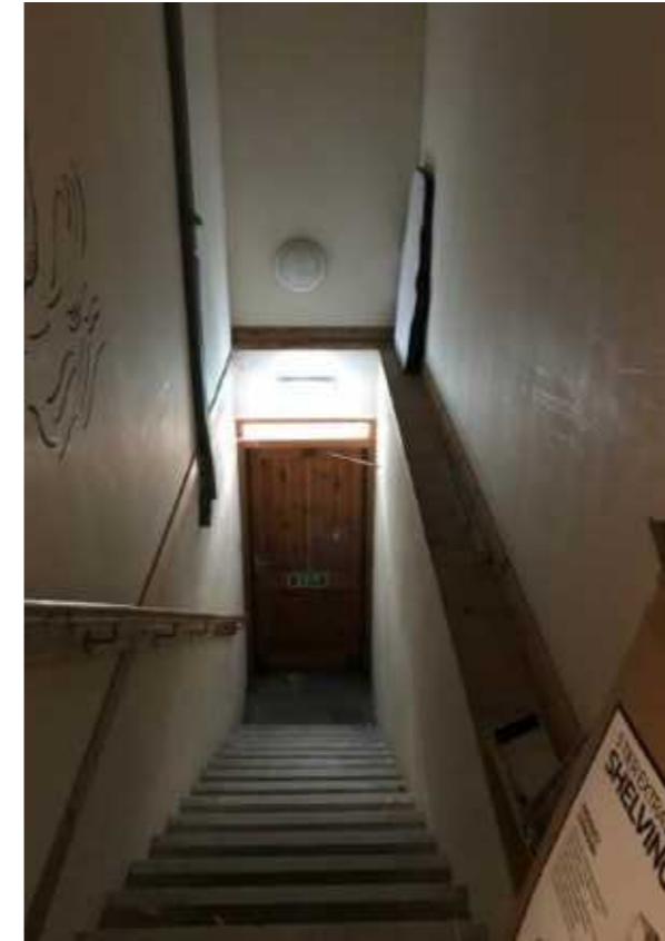
The fire exit from the gallery block the view and is inaccessible
