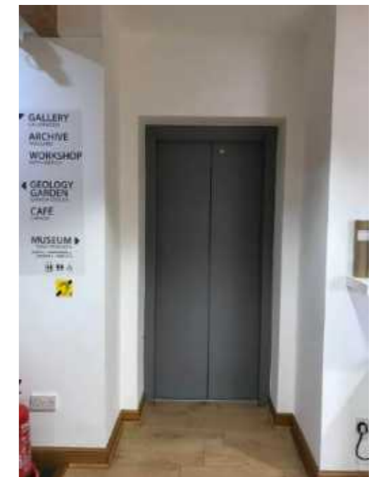
The lift access to the first floor is too small and tempermental
