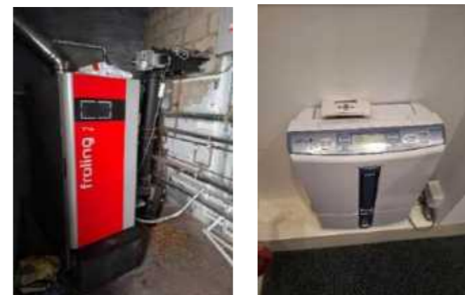
Biomass boiler and dehumidifier
