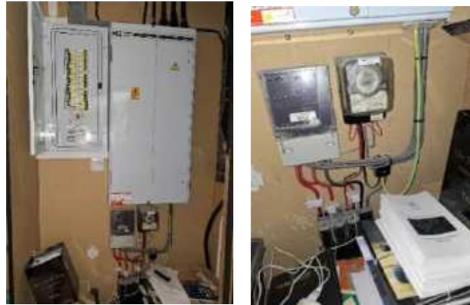
Existing electrical incomer and main DB
