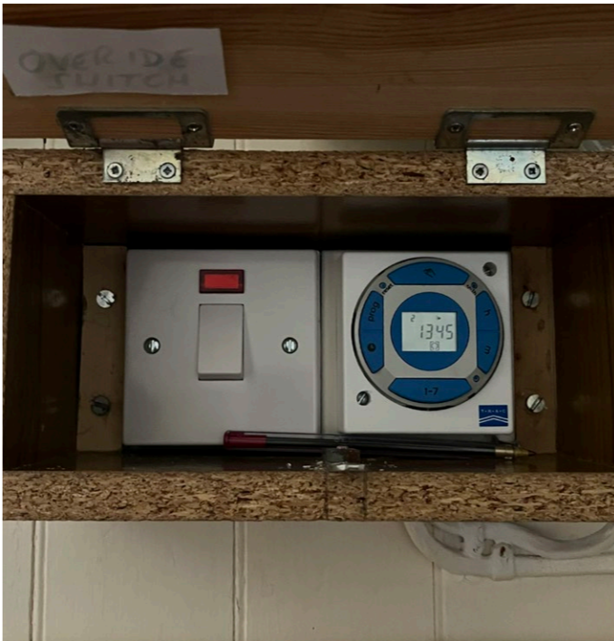
Override switch for the heating in the Vestry
