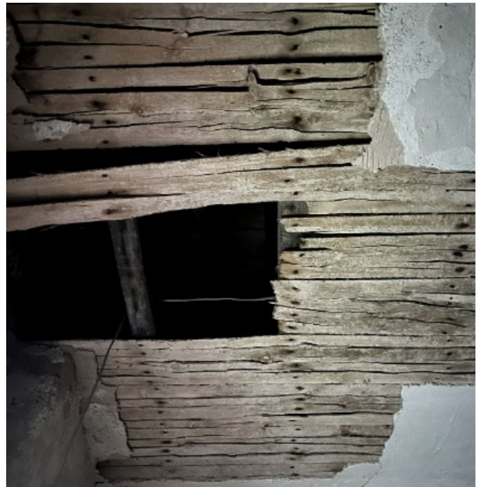
Original lath and plaster ceiling above the newer suspended ceiling of the Parish Hall
