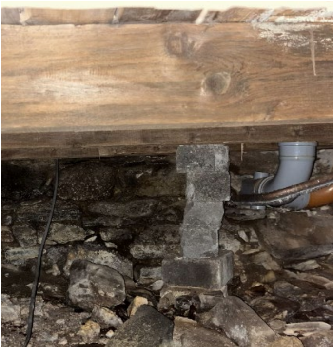
Subfloor below the WC
