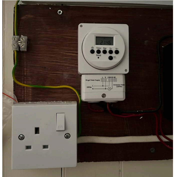
Thermostat for the heating in the Vestry
