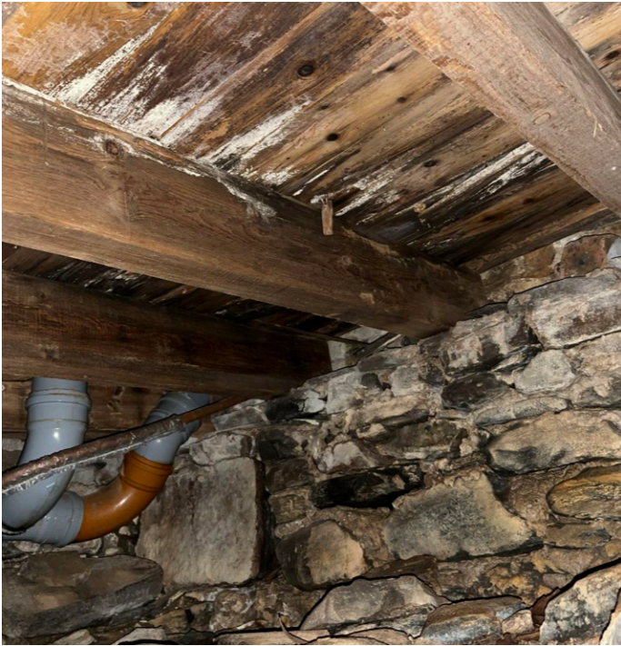
Foul drainage below the WC
