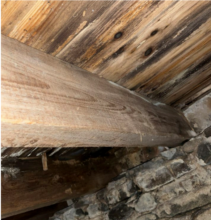
Subfloor below the WC
