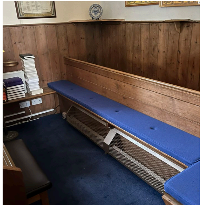
Electric heaters below the pews in the Nave
