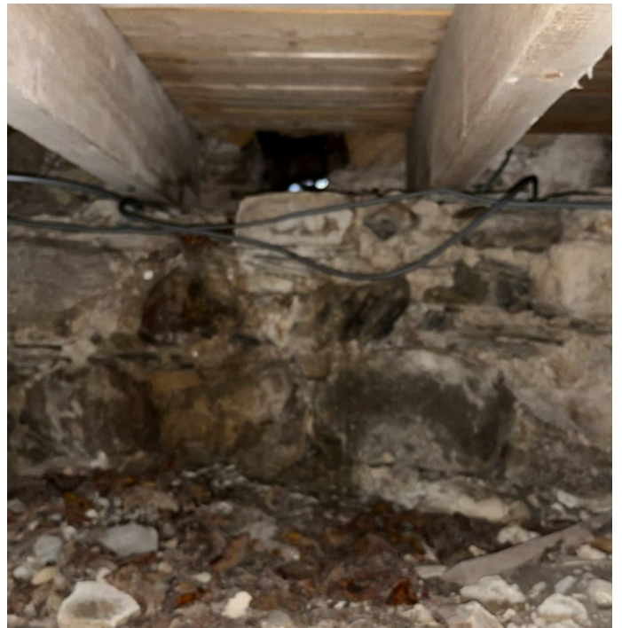
Solum vent blocked with steel mesh to prevent rodent access (28.10.2025)
